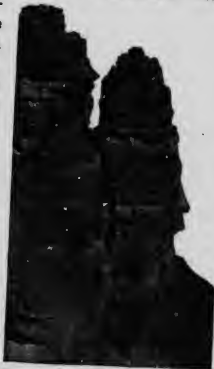
FIG. 35. — Weathered sandstone. The rock is composed of horizontal layers, and is divided by vertical joints. The weathering is most rapid along joints and at the divisions between layers.
